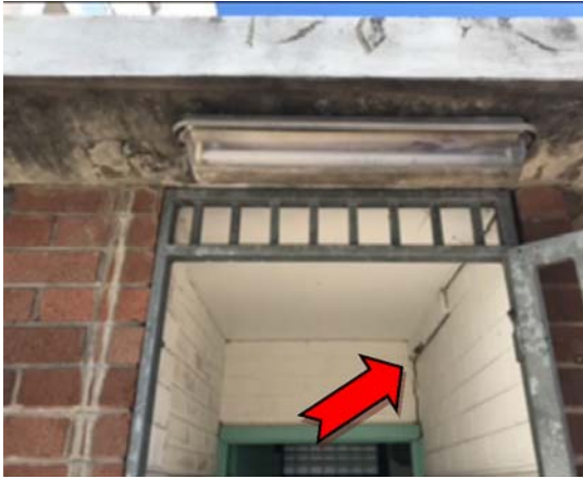
Photo 1. Exterior, entrance to state transit room, to wall, expansion joint – non-friable asbestos-containing bituminous material.
